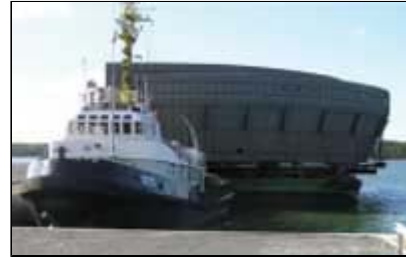
On July 15, the first sections of metallic liner for the inside of the reactor containment building arrived by the sea at the Olkiluoto 3 construction site.
