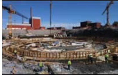
Summer 2005: Situation on site looking at the basemat of the reactor building
